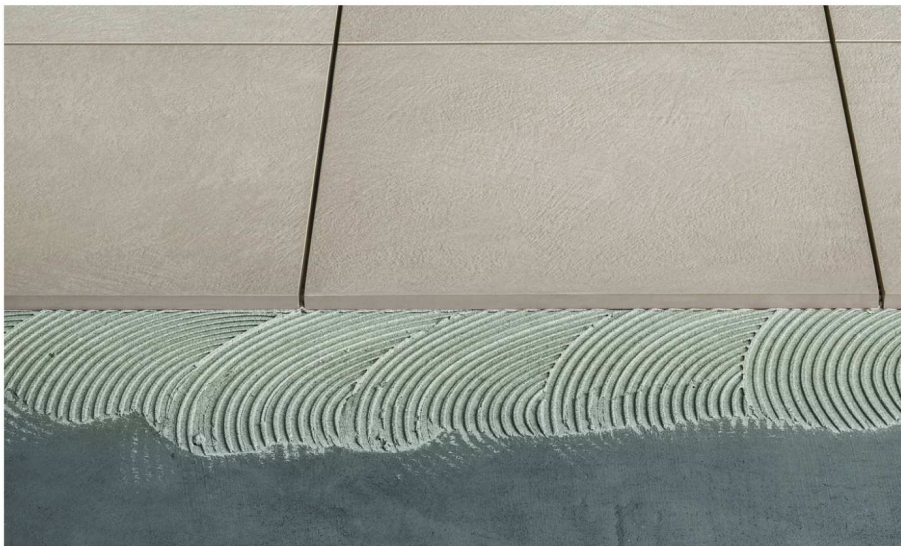
Laying 1cm tiles with tile adhesive onto an existing concrete substrate (will require grouting)
